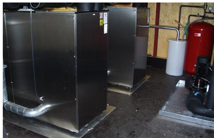
Photo. 4: Two indoor Hydro-Carbon chillers.
