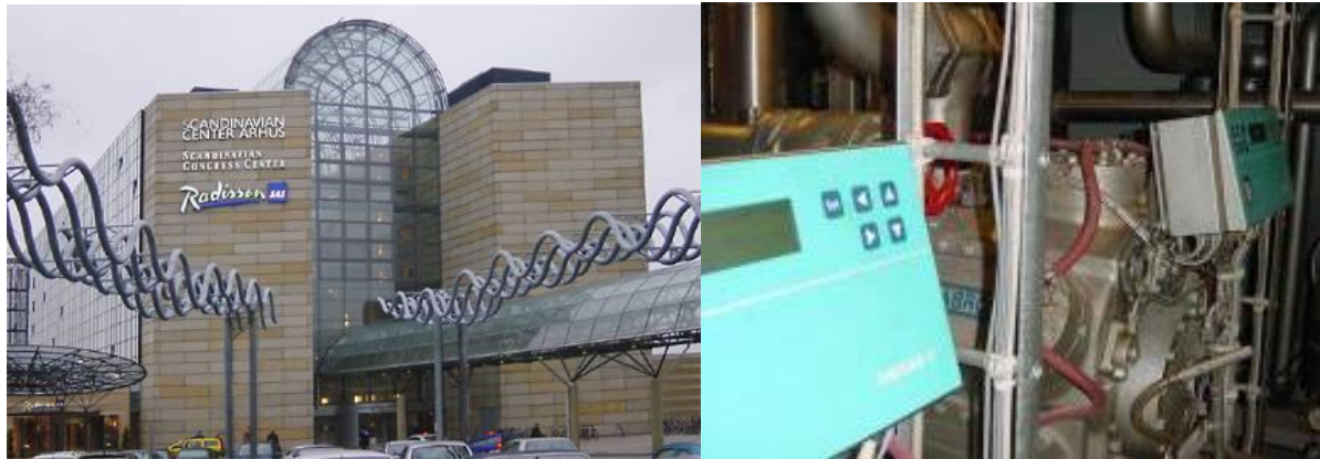
Photo. 3: Scandinavian Congress Center in the center of Aarhus uses Ammonia systems with a total cooling capacity of 1,200 kW.
